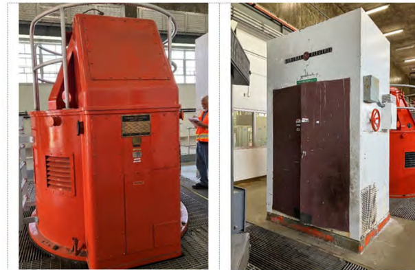
Motor and Equipment at Motor Level
