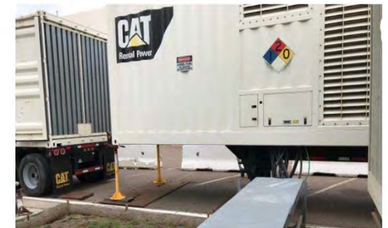
Temporary Power Generator at PS2
