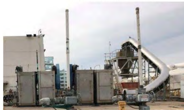
Aboveground Screens and Conveyor
