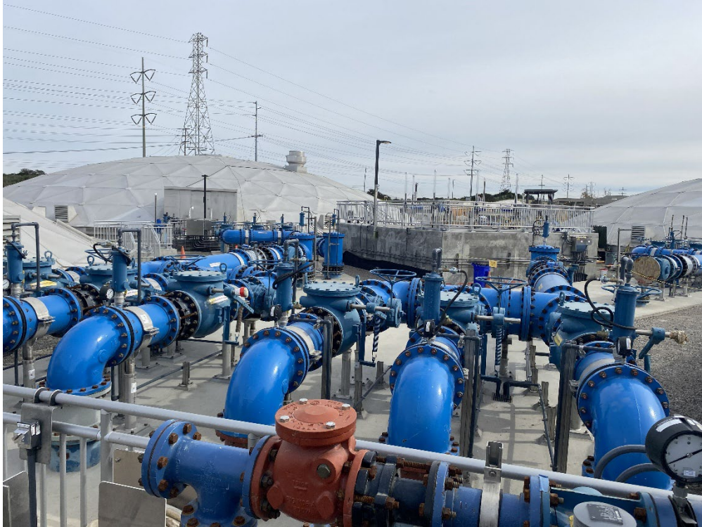
North City Water Reclamation Plant Pure Water Project Secondary Clarifiers with RAS Piping (April 2026)
