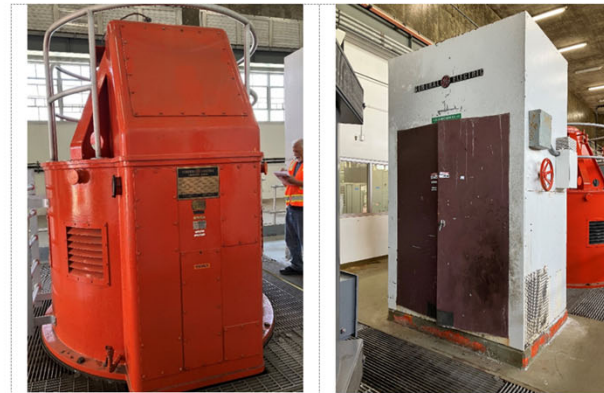
Motor and Equipment at Motor Level
