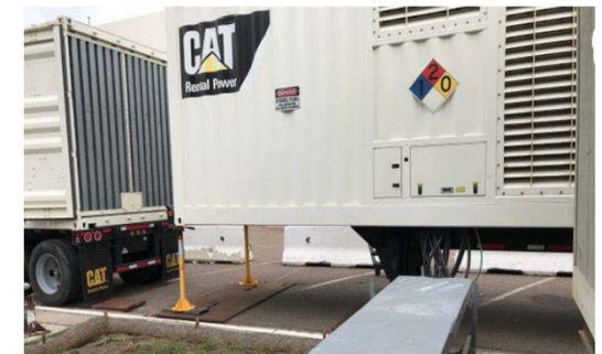
Temporary Power Generator at PS2
