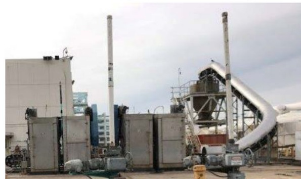
Aboveground Screens and Conveyor
