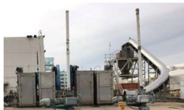
Aboveground Screens and Conveyor
