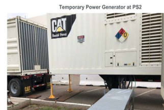
Temporary Power Generator at PS2
