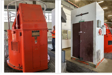
Motor and Equipment at Motor Level
