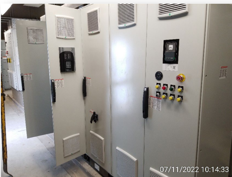
Photo 3. The new installed VDF.
