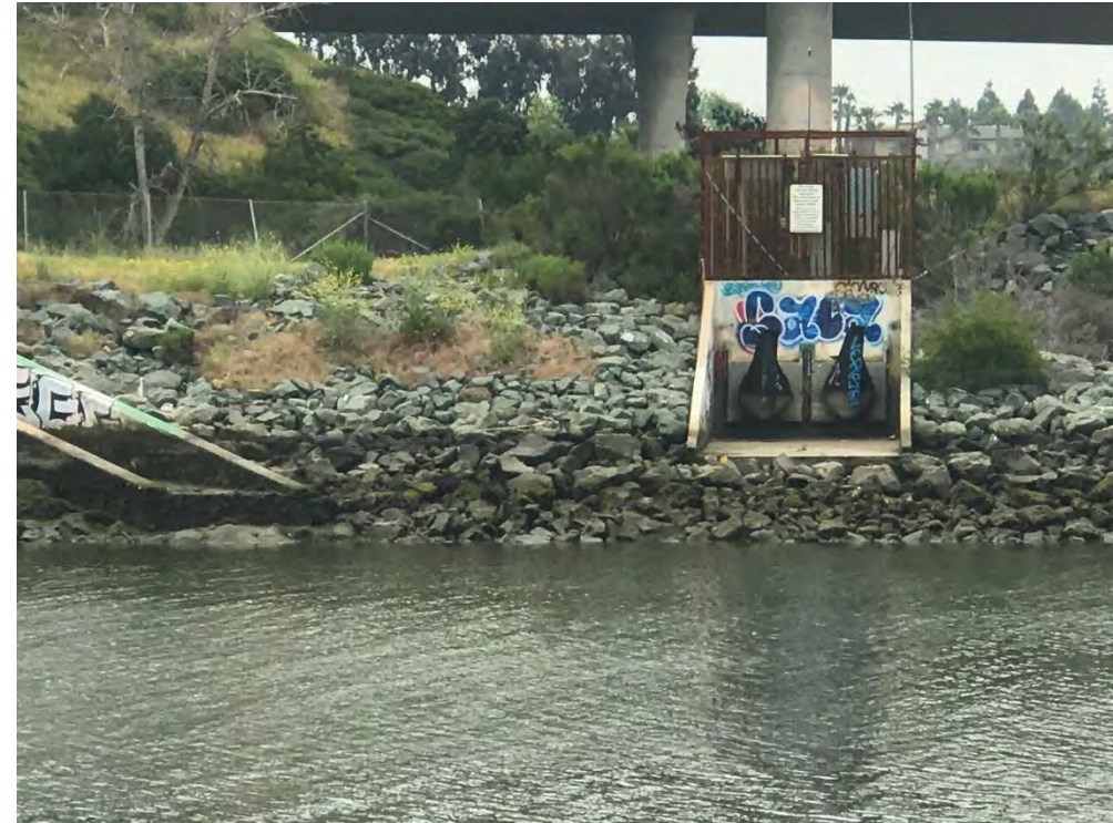
South Siphon Transition Structure
