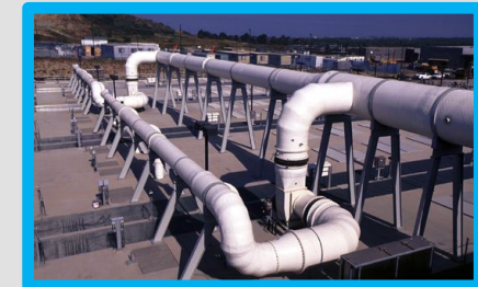
South Bay Water Reclamation Plant
