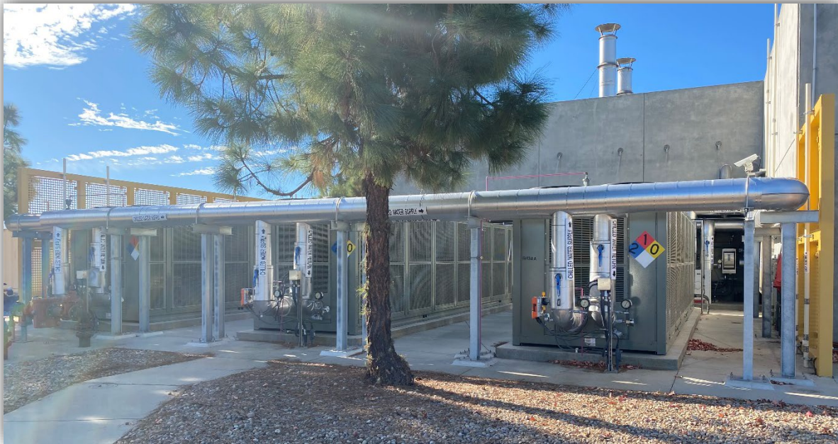
Three (3) new 250-Ton chiller units
