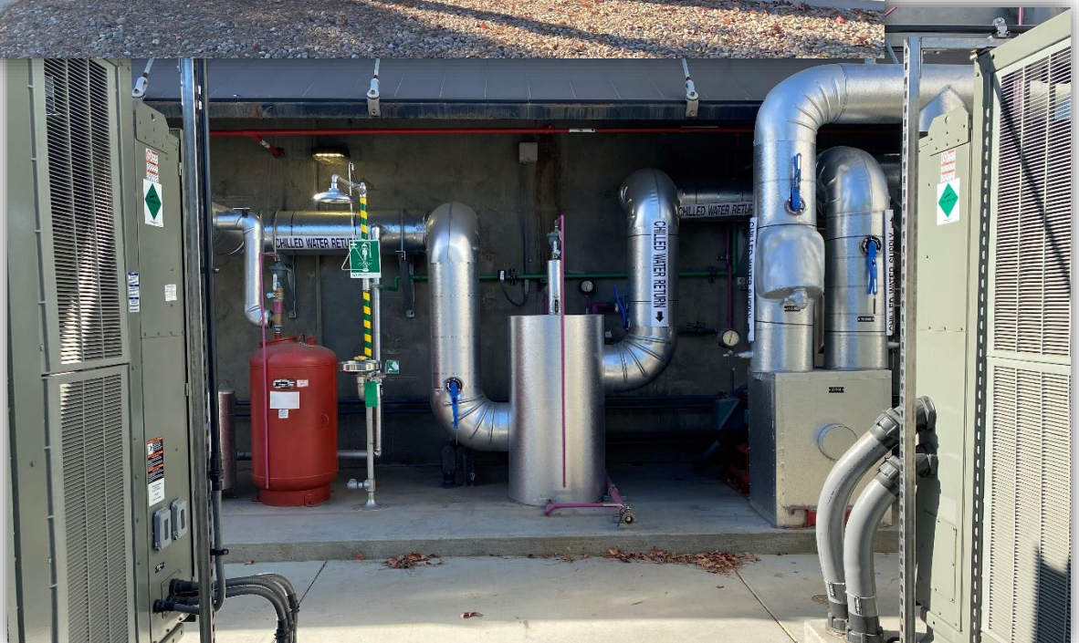
New chemical and air separator tanks
