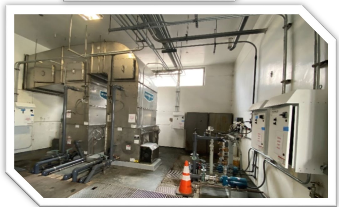
Photo 3. PS1 New cooling towers and pumps.
