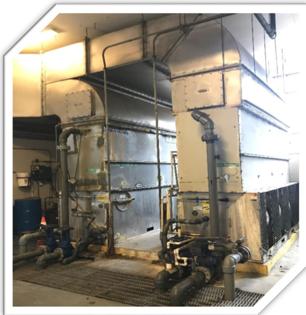
Photo 4. PS2 Existing cooling towers.
