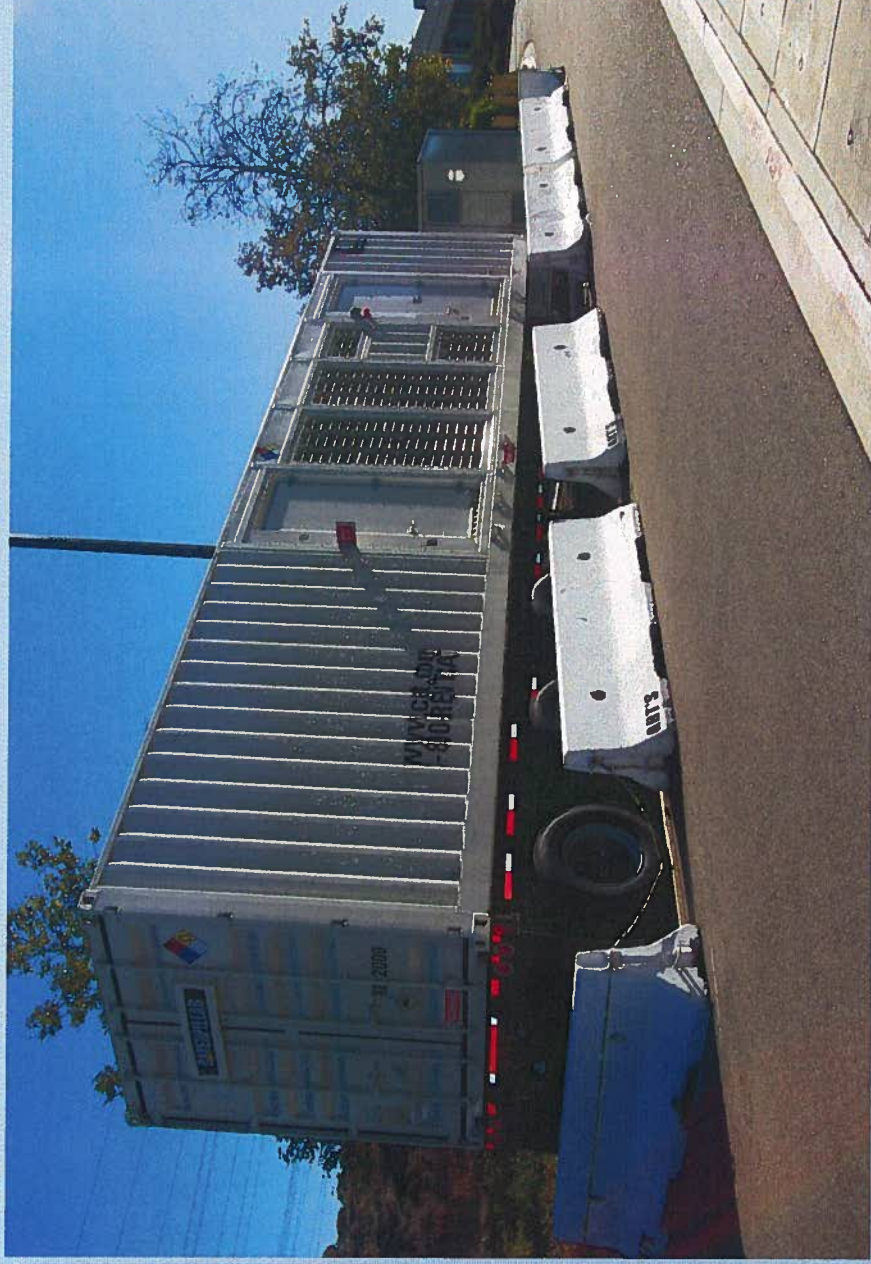
2MW Generator and transformer at North City Water Reclamation Plant
