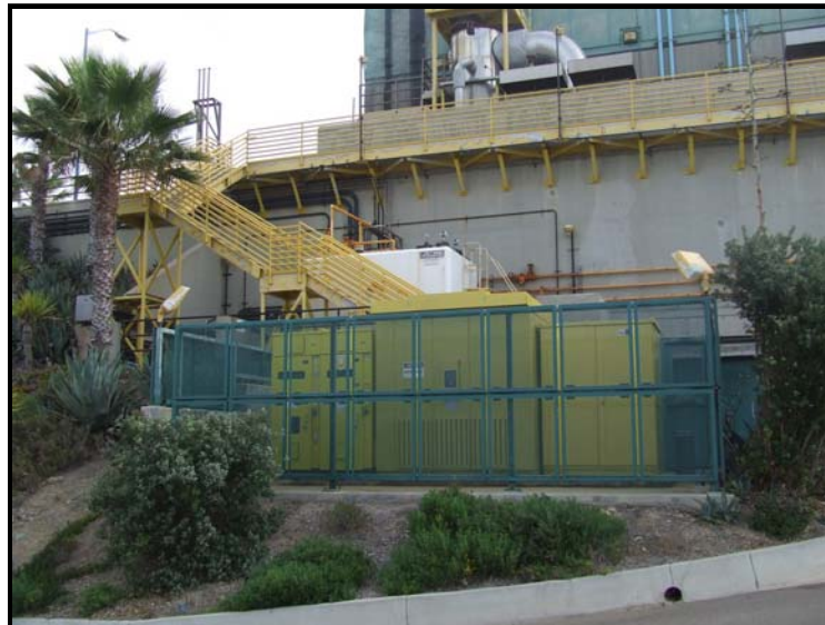
Point Loma Wastewater Treatment Plant
